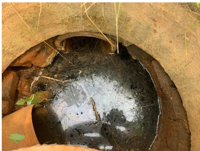
CB - 2 (Catch Basin)
