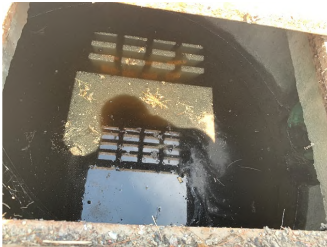
CB - 1 (Catch Basin)
