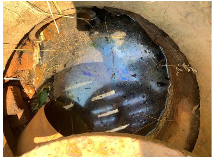
CB - 2 (Catch Basin)
