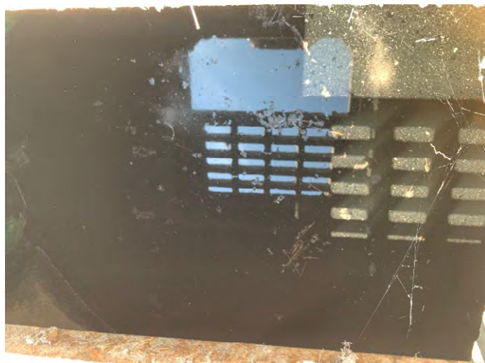
CB - 1 (Catch Basin)
