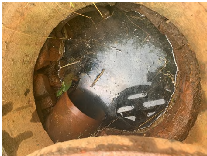
CB – 2 (Catch Basin)
