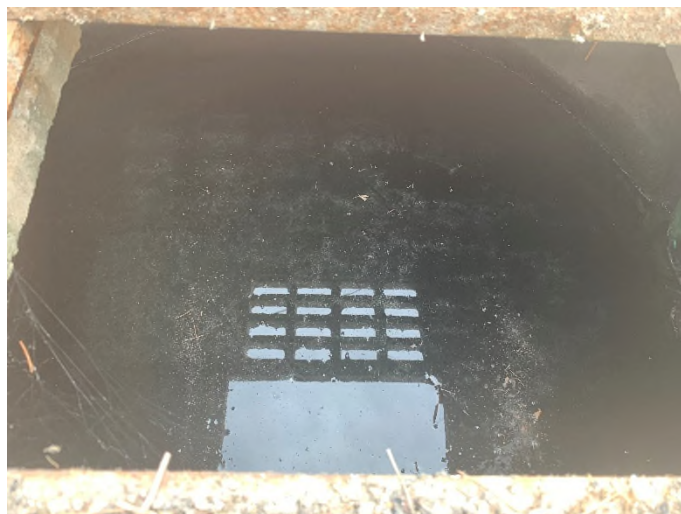
CB - 1 (Catch Basin)
