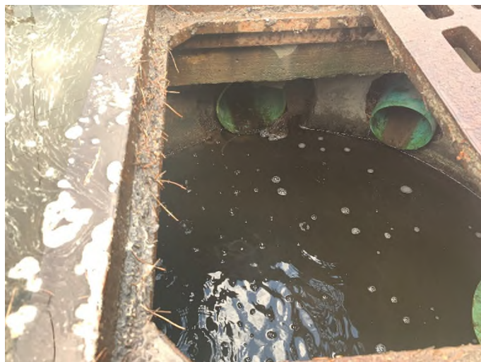
CB – 1 (Catch Basin)
