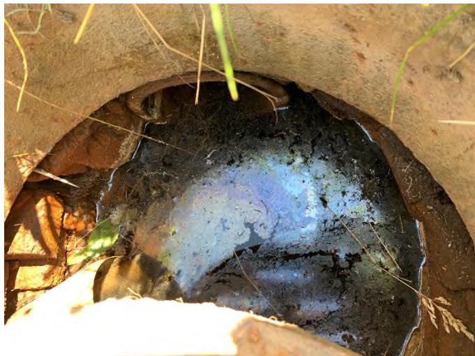
CB - 2 (Catch Basin)
