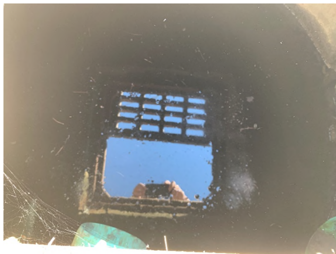
CB - 1 (Catch Basin)
