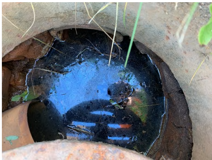
CB - 2 (Catch Basin)
